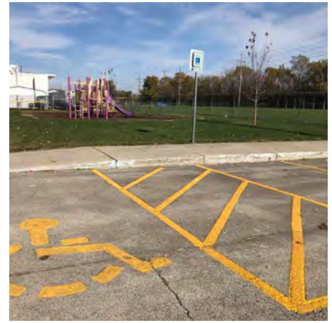
ADA parking does not meet code.
