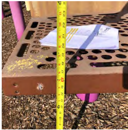
Transfer platform height meets code at approx. 17", is within the 11-18" acceptable range
