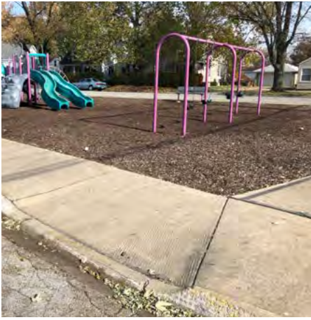
Curb ramps are not IDOT compliant a do not connect with a crosswalk
