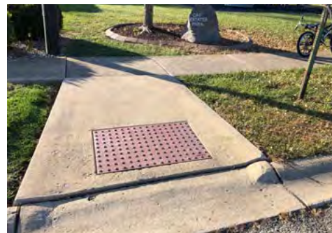
EXAMPLE OF CURB RAMP THAT DOES NOT MEET CURRENT STANDARDS, AT CAP ESTATES PARK
