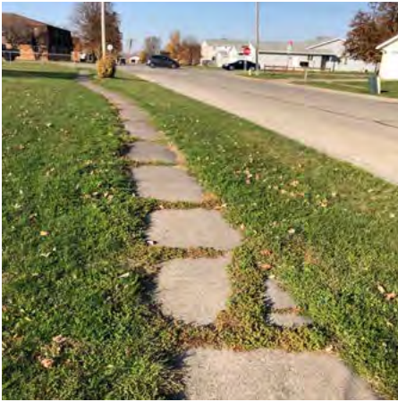
Sidewalks are too narrow at 3' wide. Joints are overgrown
