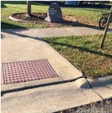
Sidewalk curb ramps are not IDOT compliant
