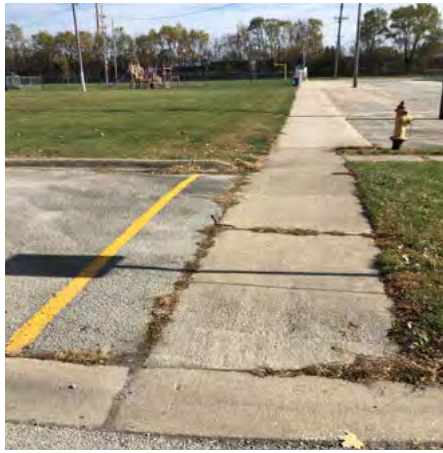
Crosswalks are not IDOT compliant
