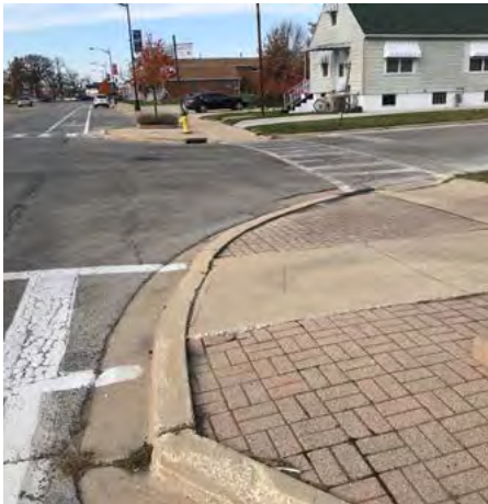
Crosswalks are not IDOT compliant
