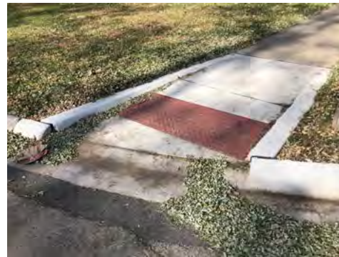
EXAMPLE OF CURB RAMP THAT MEETS CURRENT IDOT STANDARDS. NEAR FRANKLIN PARK
