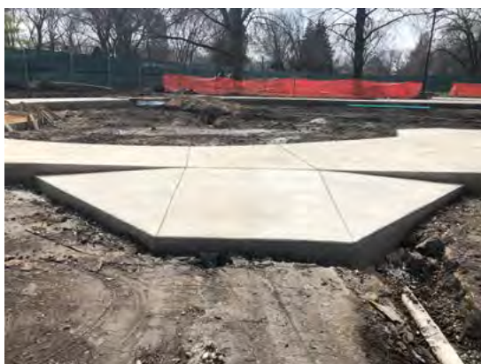
CONSTRUCTION PHOTO SHOWING A CONCRETE TRANSITION RAMP BEFORE THE SAFETY SURFACE HAS BEEN INSTALLED.
