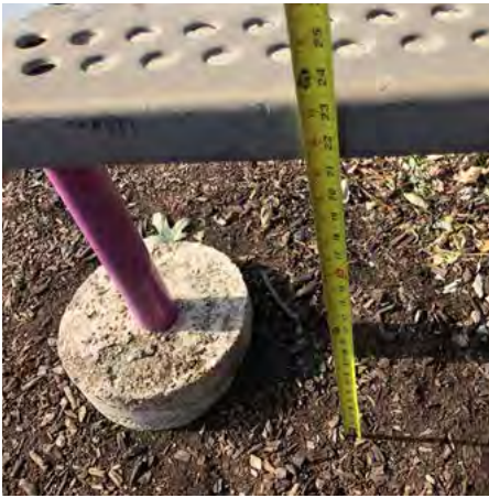
Bench in playground area. Footings are exposed and seat height is above the 19" maximum.
