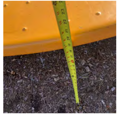
Merry-go-round does not meet safety guidelines, clear space under platform is too tall.
