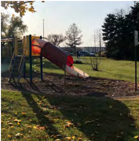
Play equipment does not meet current design standards
