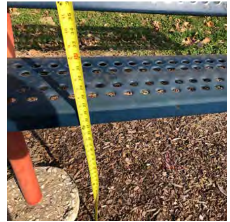
Bench in playground area. Seat height is too high, measured at approx 26", max per code is 19"
