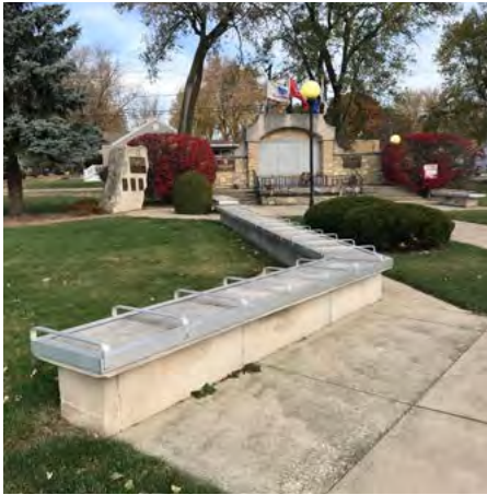
Seat walls have superficial skateboard barriers attached.
