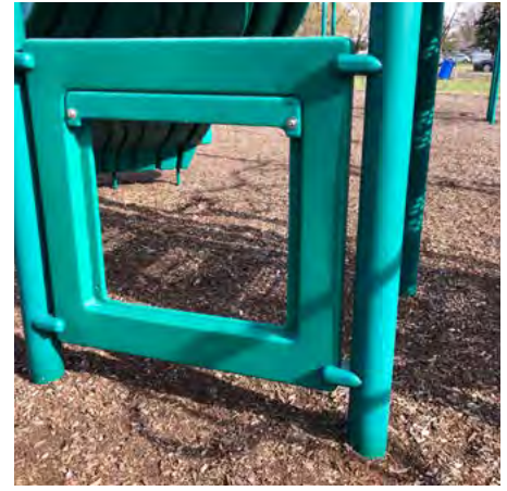
Ground level play panel has been removed.
