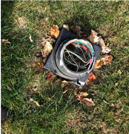
Lamp has been removed. Base and wires remain which poses a safety hazard and should be addressed
