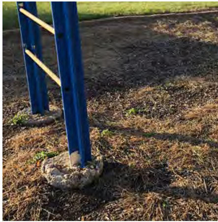
Playground equipment footings are exposed. Safety surface mulch is extremely compacted and overgrown
