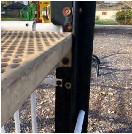
Black and White elevated component play structure has exposed and rusting fasteners
